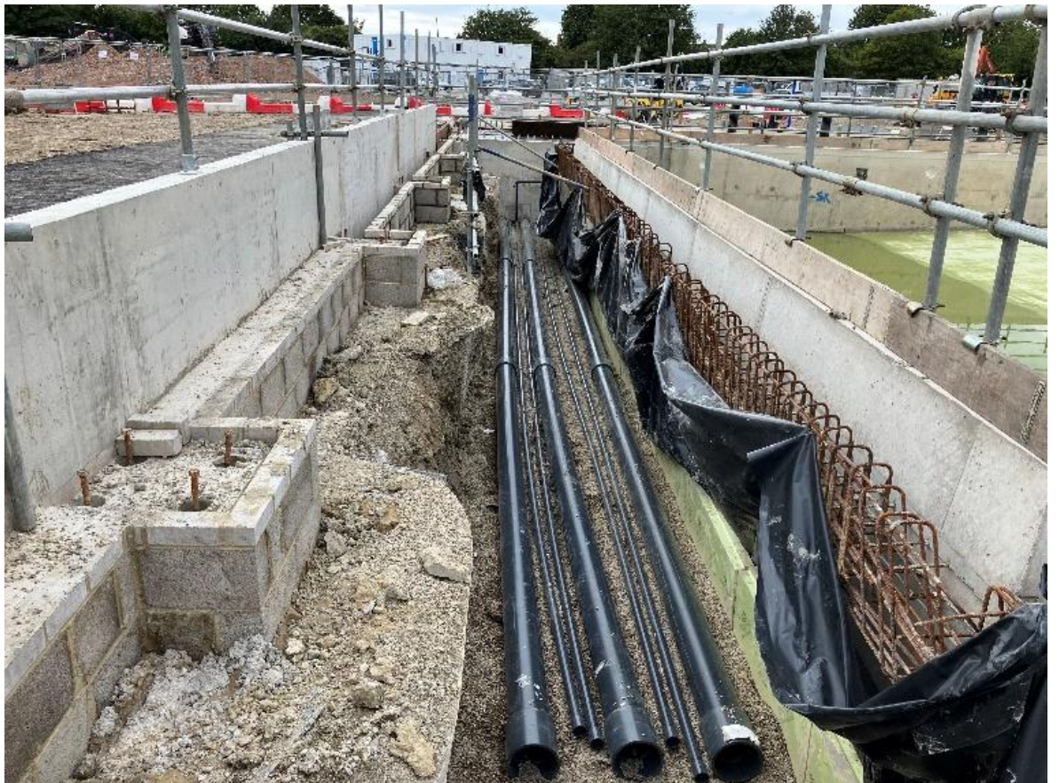
Pool Filtration Pipework
