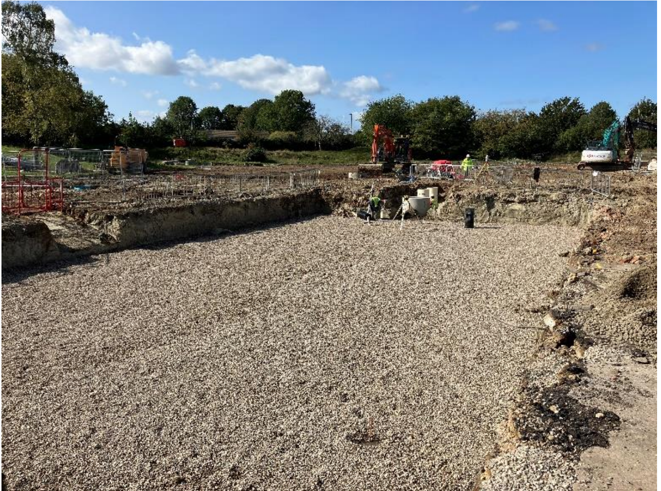
Car Park Attenuation Tank
